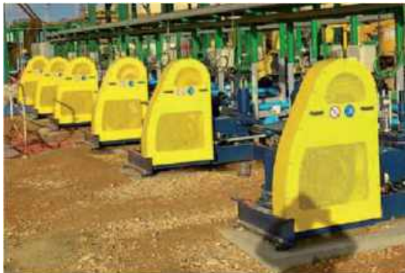
ABEL HPT gland seal water pumps on a phosphate mine in North Africa
