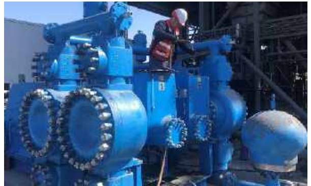
Global preventive maintenance
