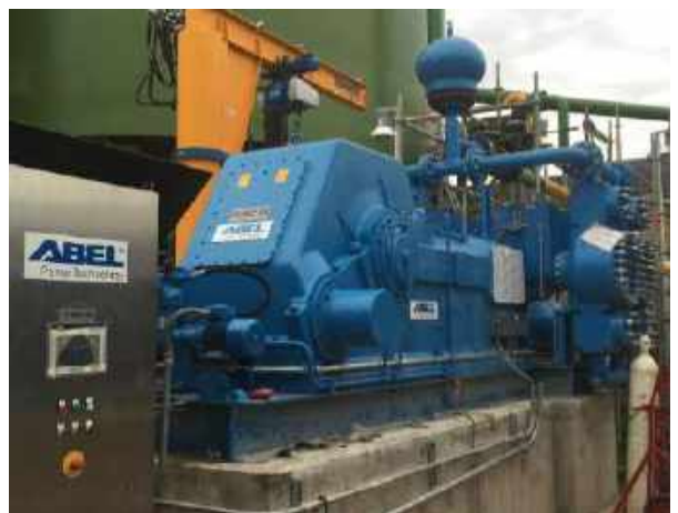
ABEL HMQ pumping paste tailings
